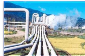
610 MW Leyte Geothermal Power Plant
