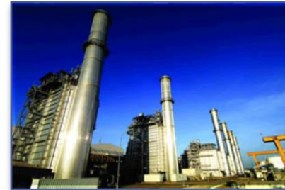
San Lorenzo Natural Gas-fired Plant
