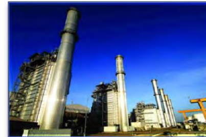
San Lorenzo Natural Gas-fired Plant
