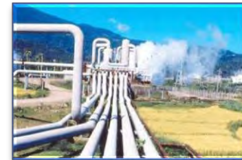
610 MW Leyte Geothermal Power Plant
