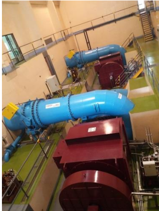
3.0MW New Bataan Hydroelectric Power Plant in New Bataan, Compostela Valley
