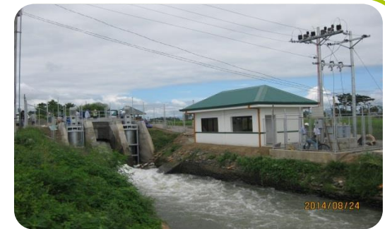
0.045MW Lateral B Hydroelectric Power Plant in San Mateo, Isabela
