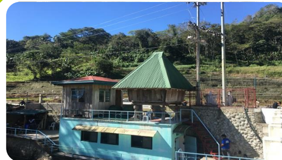
0.20MW Ambangal Hydroelectric Power Plant in Kiangan, Ifugao
