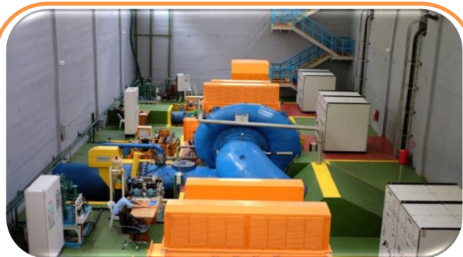
8.0MW Villasiga Hydroelectric Power Plant in Bugasong, Antique
