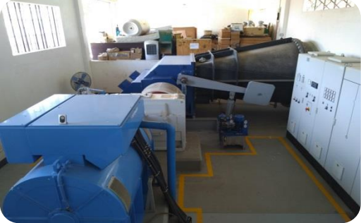
1.0MW Bulanao Hydroelectric Power Plant in Tabuk, Kalinga
