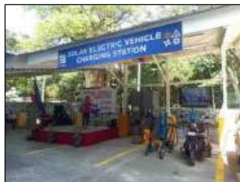
Source: UP EEEI – (AC Charger) UP Diliman, Quezon City, Metro Manila
