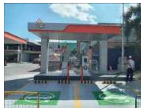
Source: Unioil EVCS – (DC Fast Charger) in Subic Bay Freeport Zone, Zambales
