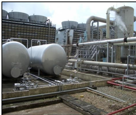
Tiwi Geothermal Power Plant (Albay)
