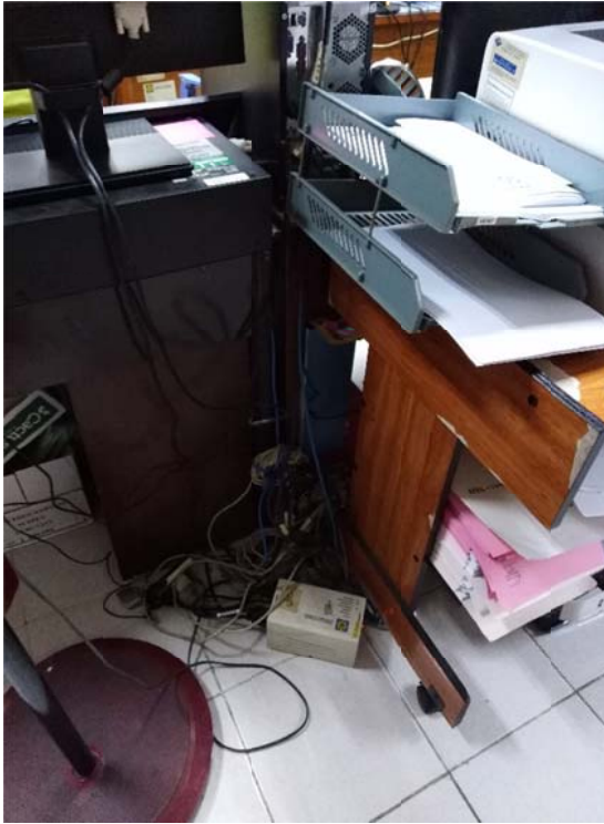
Need for proper wire management
