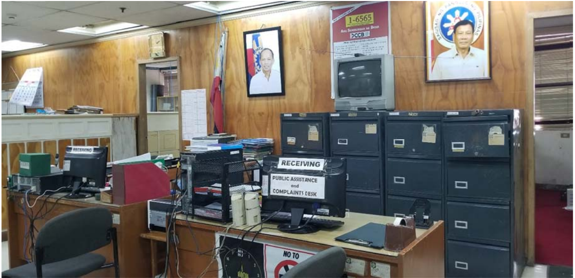
Need proper wire management of equipment
