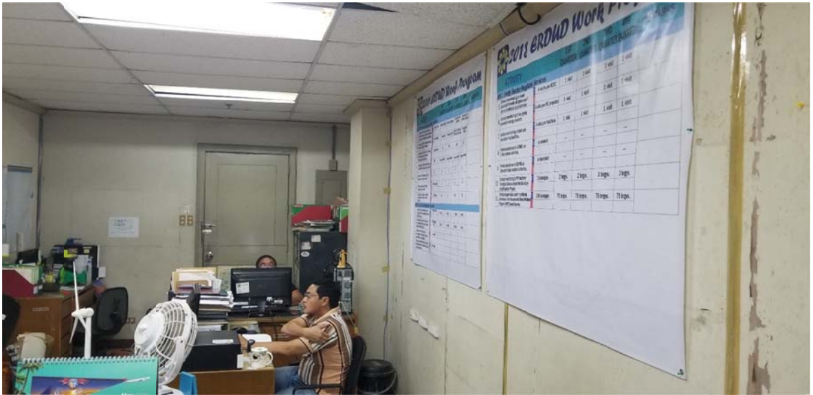
Walls need refurbishment and painting. Tarpaulins used to hide the cracks and worn-out walls
