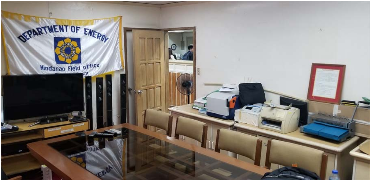
Wall cracks and big holes in the conference was hidden with a big banner. The conference hall need to be improved since it also serves as storage of other office equipment
