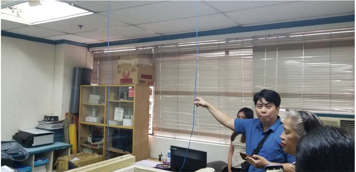
Need proper IT wire management of internet connection
