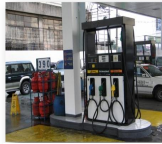
Figure 3. Pump in a gas station
